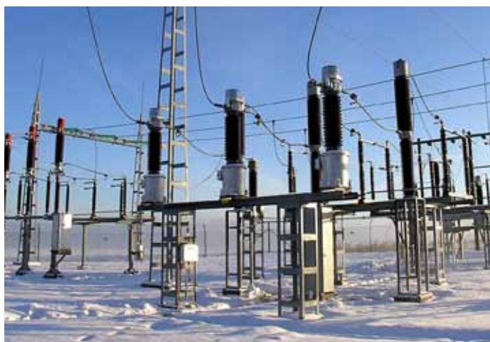
Substation in Sweden with cold climate. ABB equipment with IMB 145.
