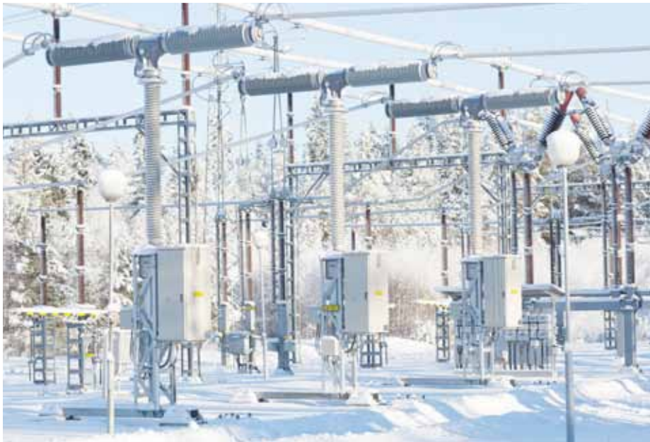
FOCS integrated in the top of a 420 kV circuit breaker
