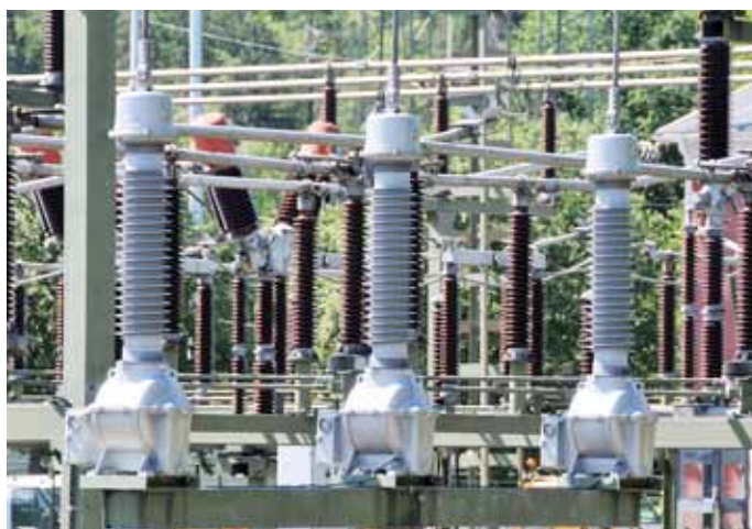
Inductive voltage transformers EMF 145. Installed in Sweden.
