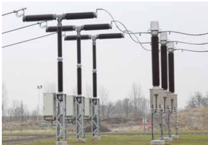
LTB 420 E2 with current transformer IMB 420. Installation in Denmark.
