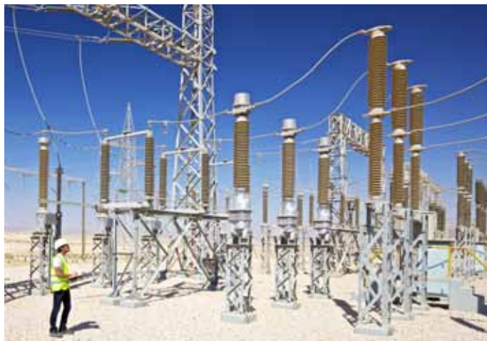
Substation in Oman with desert climate. ABB equipment with IMB 145.
