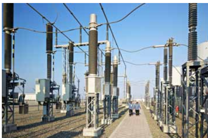
Substation in Oman with desert climate. ABB equipment with IMB 245.
