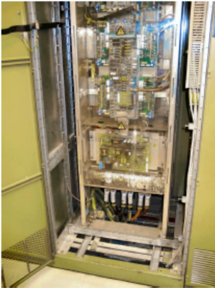
Pic 8. SAFUI inverter unit in MX cabinet
