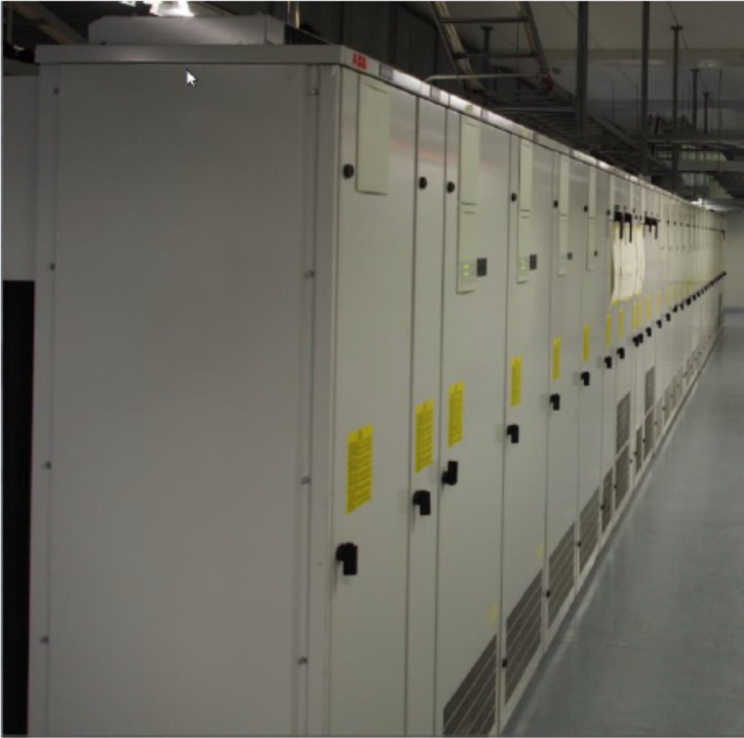
Pic 31. ACS600 multidrive cabinet line-up
