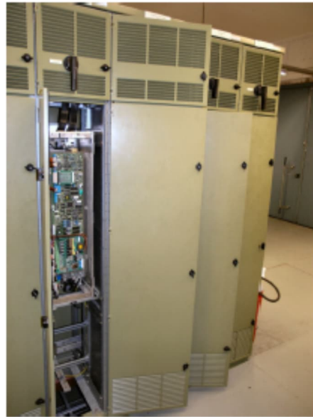
Pic 9. MX cabinet, drive sections
