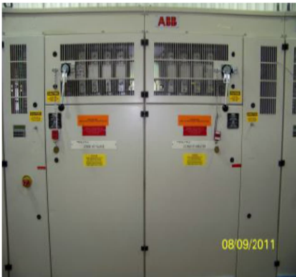
Pic 29. Nema cabinet line-up
