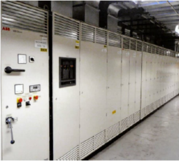
Pic 14. MD cabinet line-up
