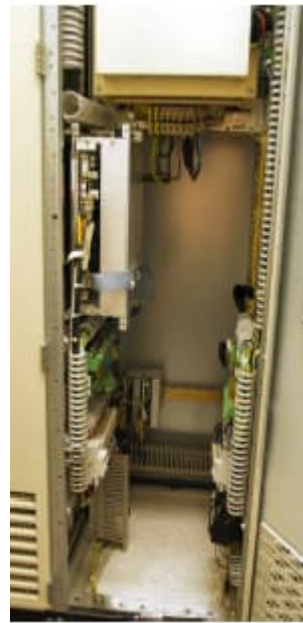
Pic 37. APC rack, 1 empty slot available.
